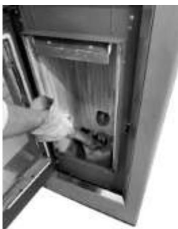
Fig. 33 - Burning pot box cleaning
